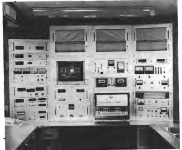
Fig. 1.55 – Example well monitoring unit.
